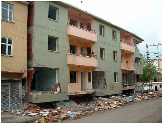
Gambar 2. Soft-storey - Gempa Bingol, Turki 2003
